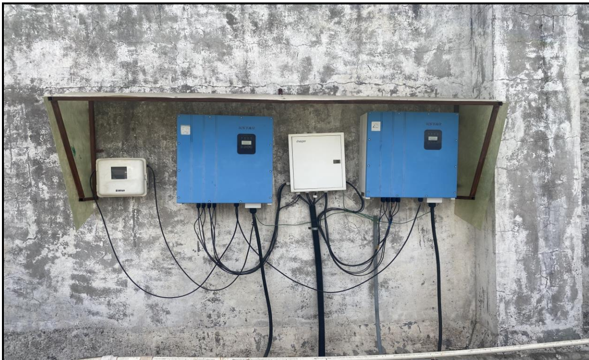
Figure 3.1:- Solar Plant 480 KWp and Inverter System
